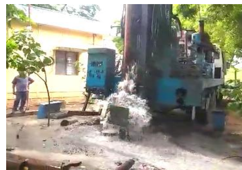
Well drilled by CGWB at Pallamale village in Chimakurthy block of Prakasam district, Andhra Pradesh.
