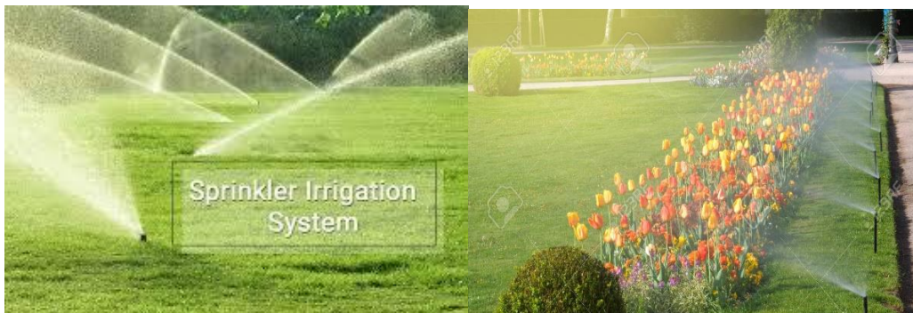
(i) Sprinkler system in different farm lands (ii) Automatic Sprinkler system in the garden
