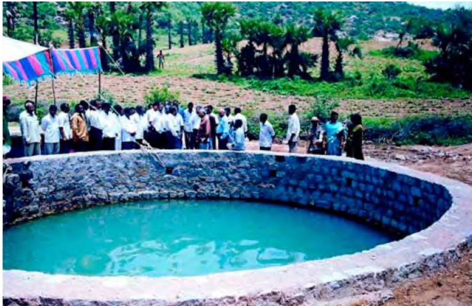
Fig 14 Capture well rejuvenated by recharged water
