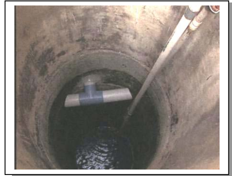
Abandoned Dug Well fitted with Rain Water Harvesting Mechanism
