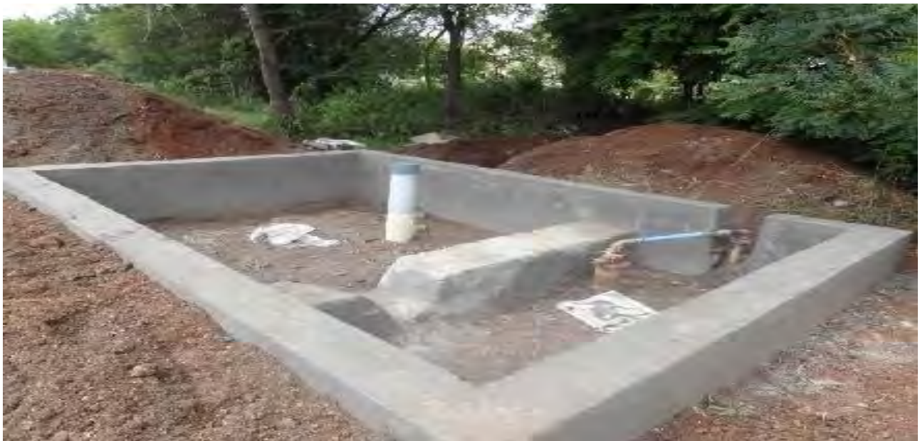
Recharge Pit with Existing Bore Well
