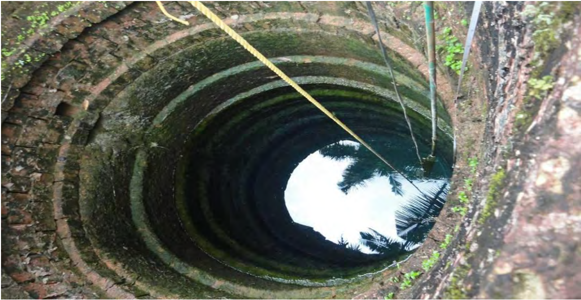
A View of Observation well after the construction of AR structures in the School campus
