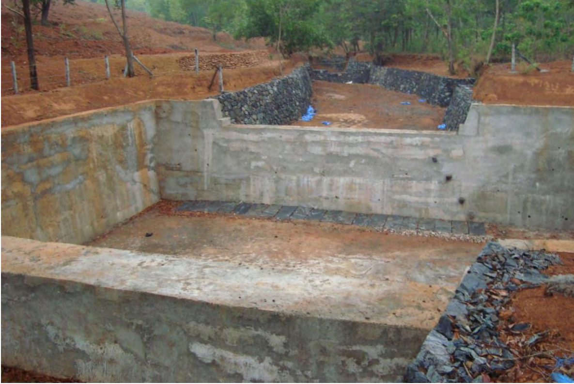
Recharge Pond with Check Dam in the middle reaches of the main stream
