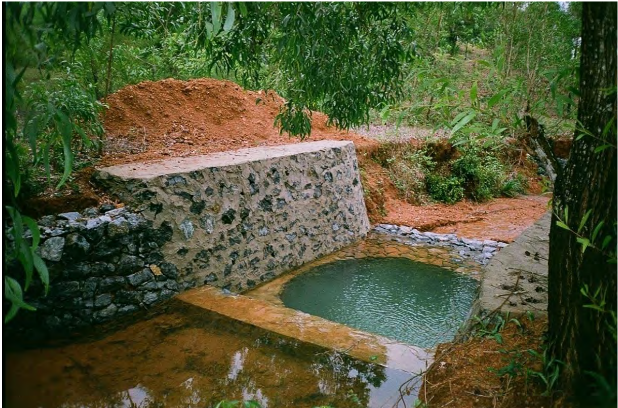
A view of the Circular Recharge Pit filled with water
