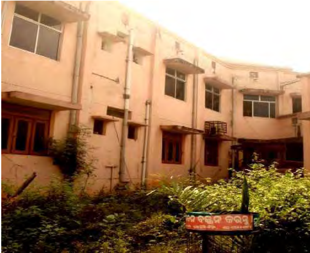
COLLECTION PIPE LINES ON BACK SIDE OF DRDA OFFICE BUILDING, COLLECTORATE CAMPUS, KHURDA DIST.
