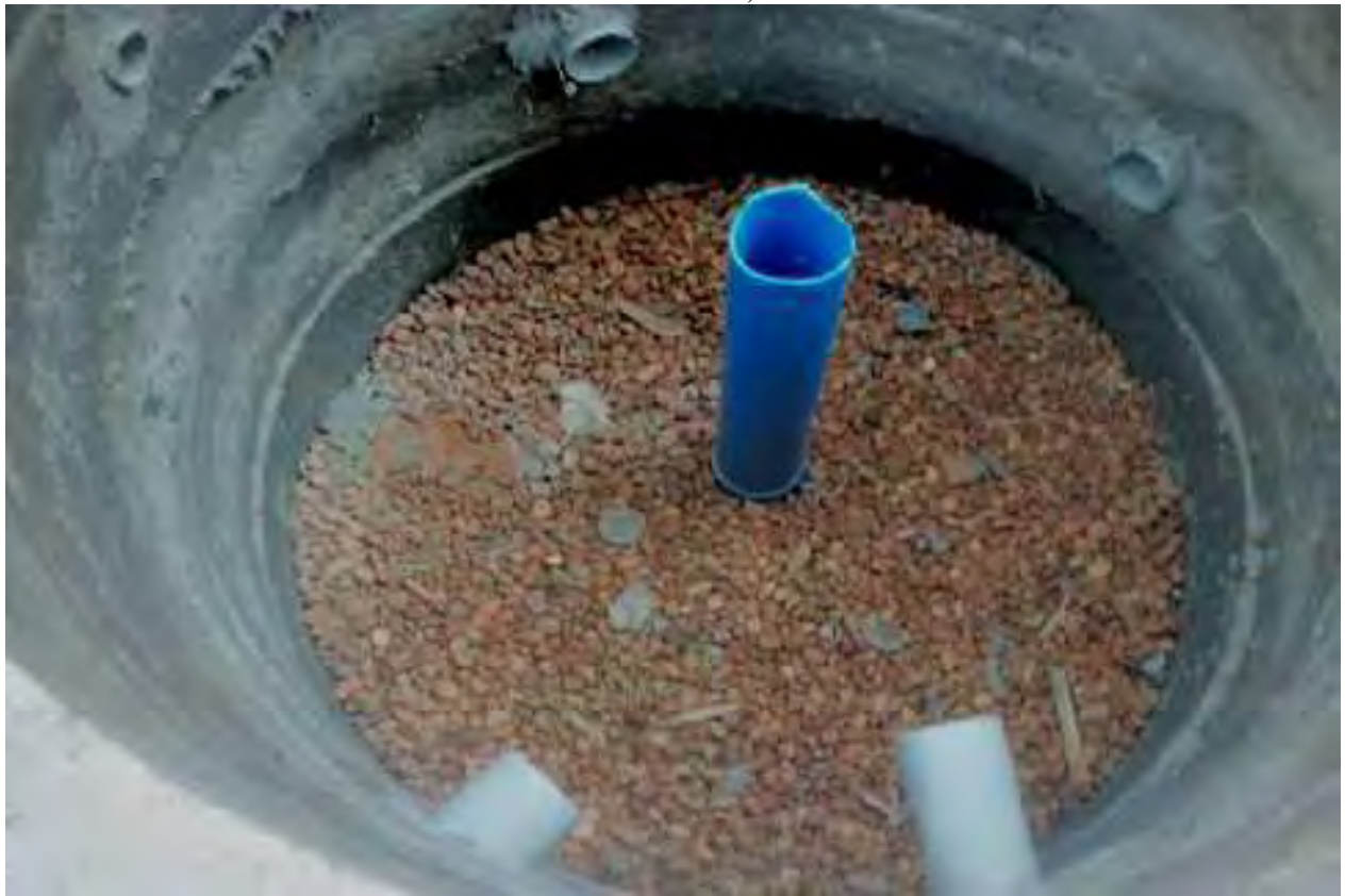
[RECHARGE BORE WELL] OFFICE BUILDING, COLLECTORATE CAMPUS, KHURDA DIST
