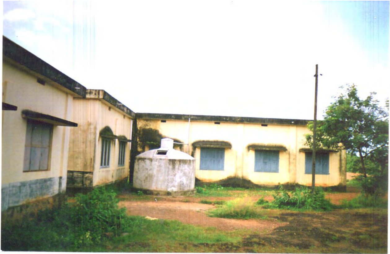
A view of the Ferrocement Tank Artificial Recharge in Kolathur-II, Bedadka Grama Panchayat, Kasargod, Kerala
