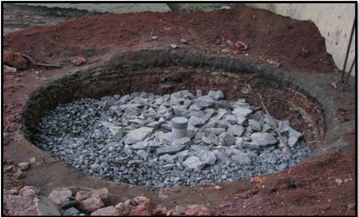
Circular Structure RWHS in Coimbatore city, Coimbatore Block, Dist. Coimbatore, Tamil Nadu
