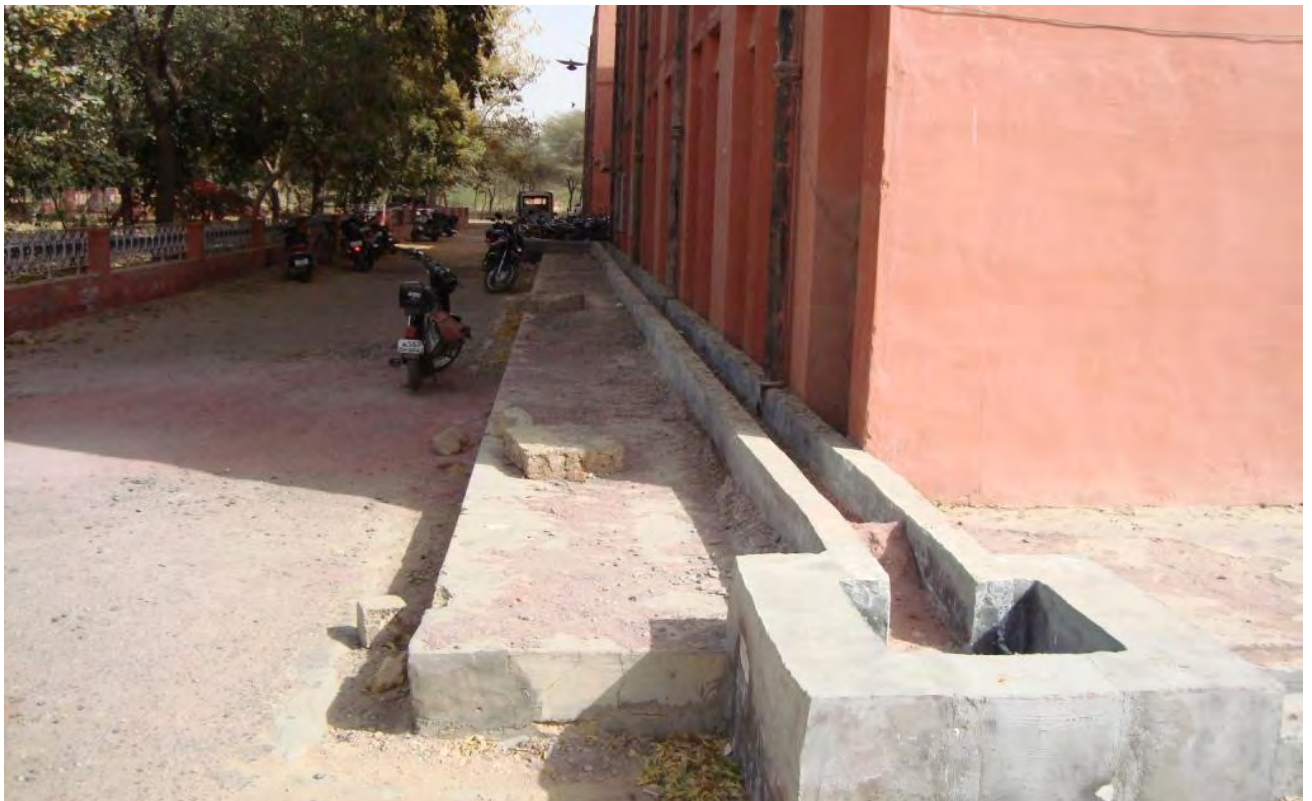
Water Channel for collection of roof top runoff-CE, IGNP Office Building, Bikaner city, Dist Bikaner
