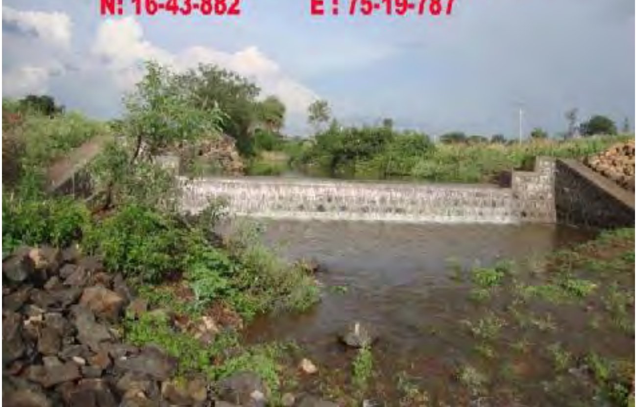
Check dams constructed in the sub watershed, Arthal Water Shed Artificial Recharge in Arthal Water Shed, Athni Block Belgavi District, Karnataka
