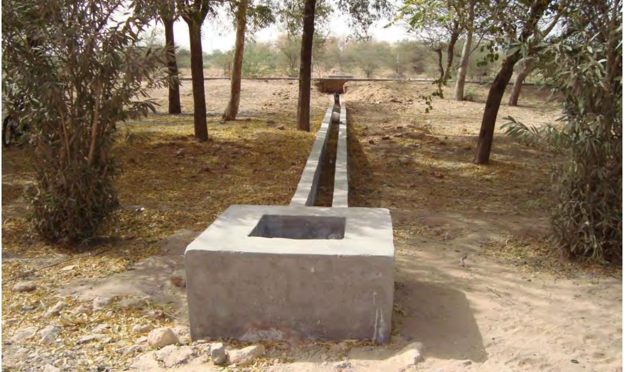
Water Channel with siphon pit-CE, IGNP Office Building, Bikaner city, Dist Bikaner
