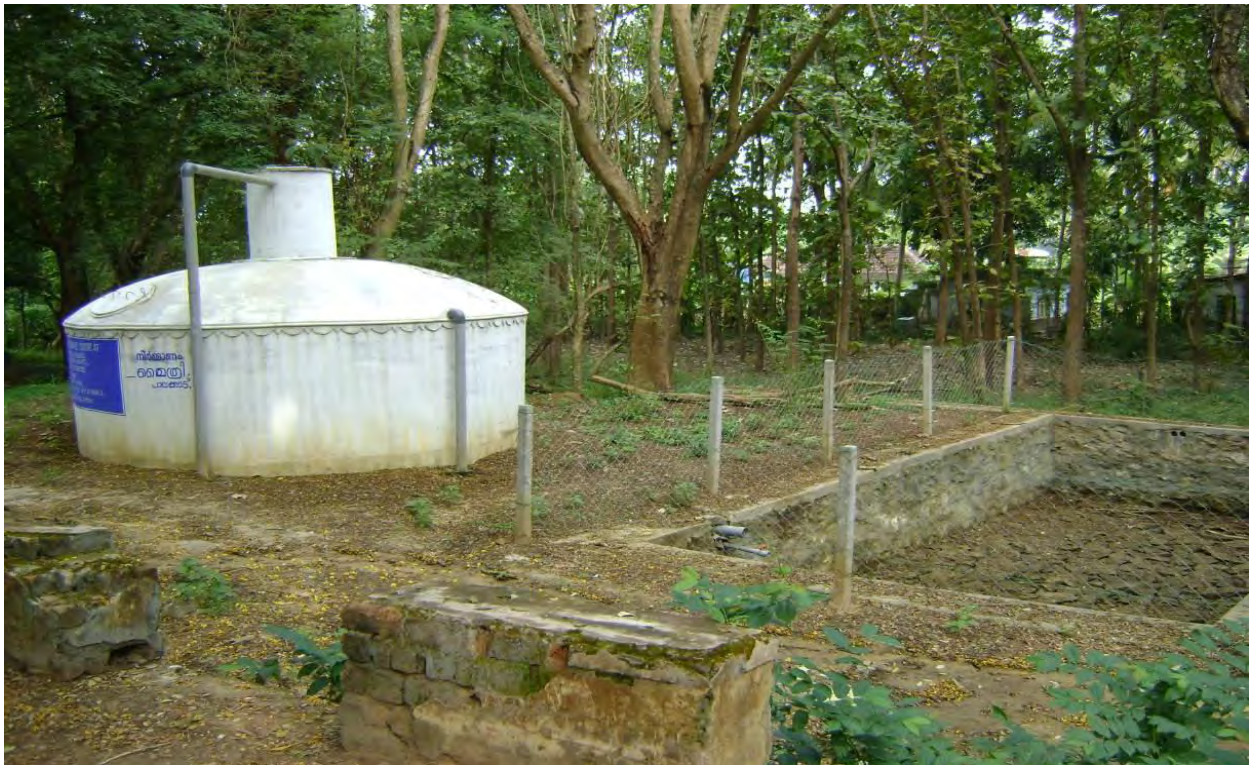
Roof Top Rain Water Harvesting at Govt. college, Chittordist, Kerala
