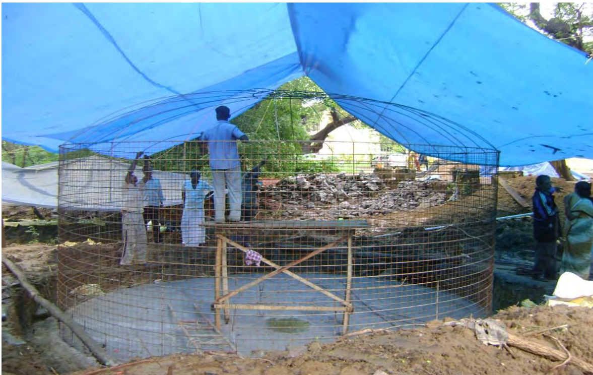
Ferro Cement Tank under construction Roof Top Rain Water Harvesting at Govt. college, Chittordist, Kerala
