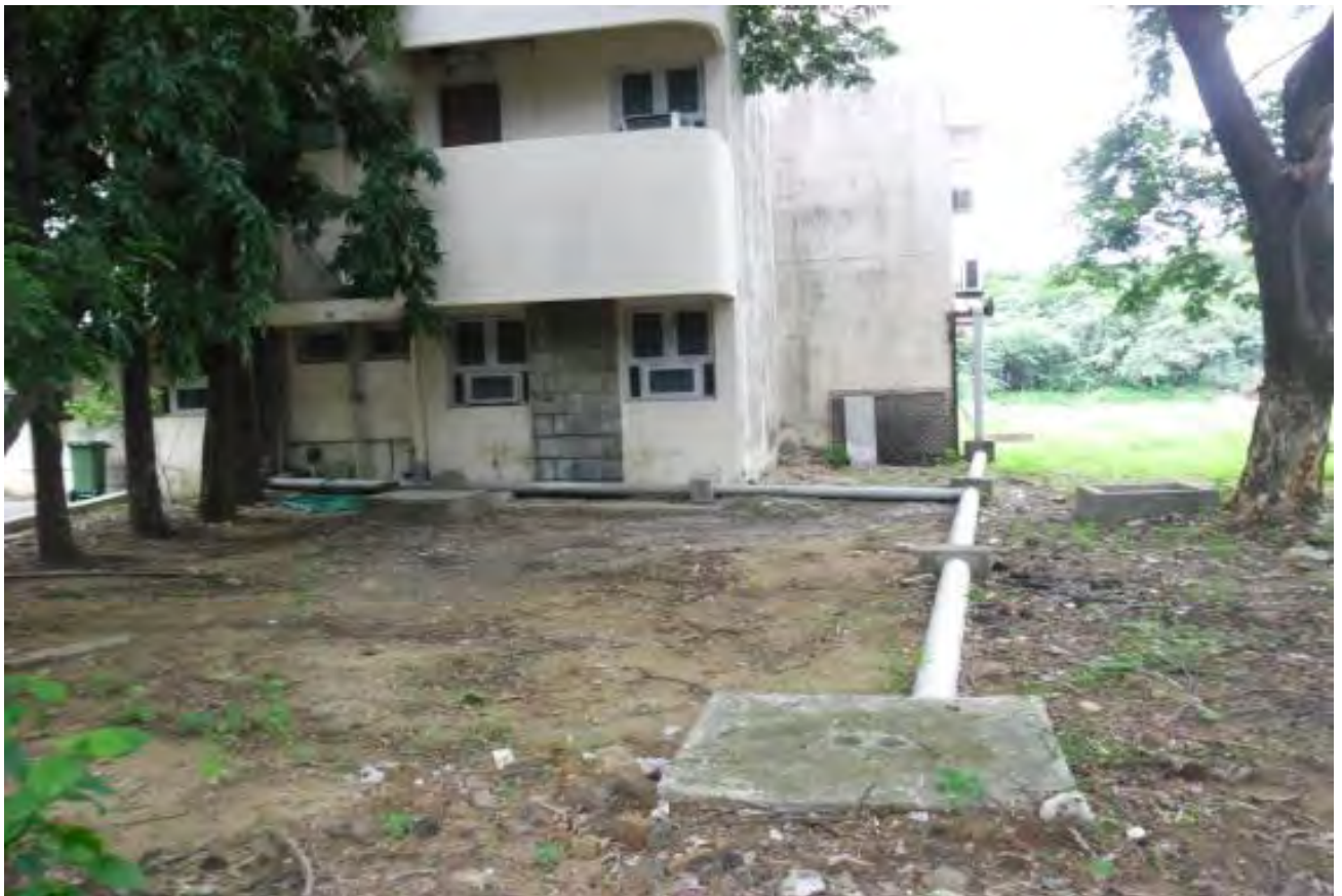
Collection, conveyance and Filtering Unit of roof top rainwater harvesting Rain water Harvesting in the premises of the NITTTR, Taramani, Chennai city, Tamil Nadu.
