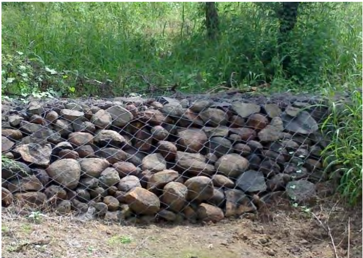
Gabion Structure-After monsoon Artificial Recharge to Groundwater in Raj Bhawan area, Nagpur, Maharashtra
