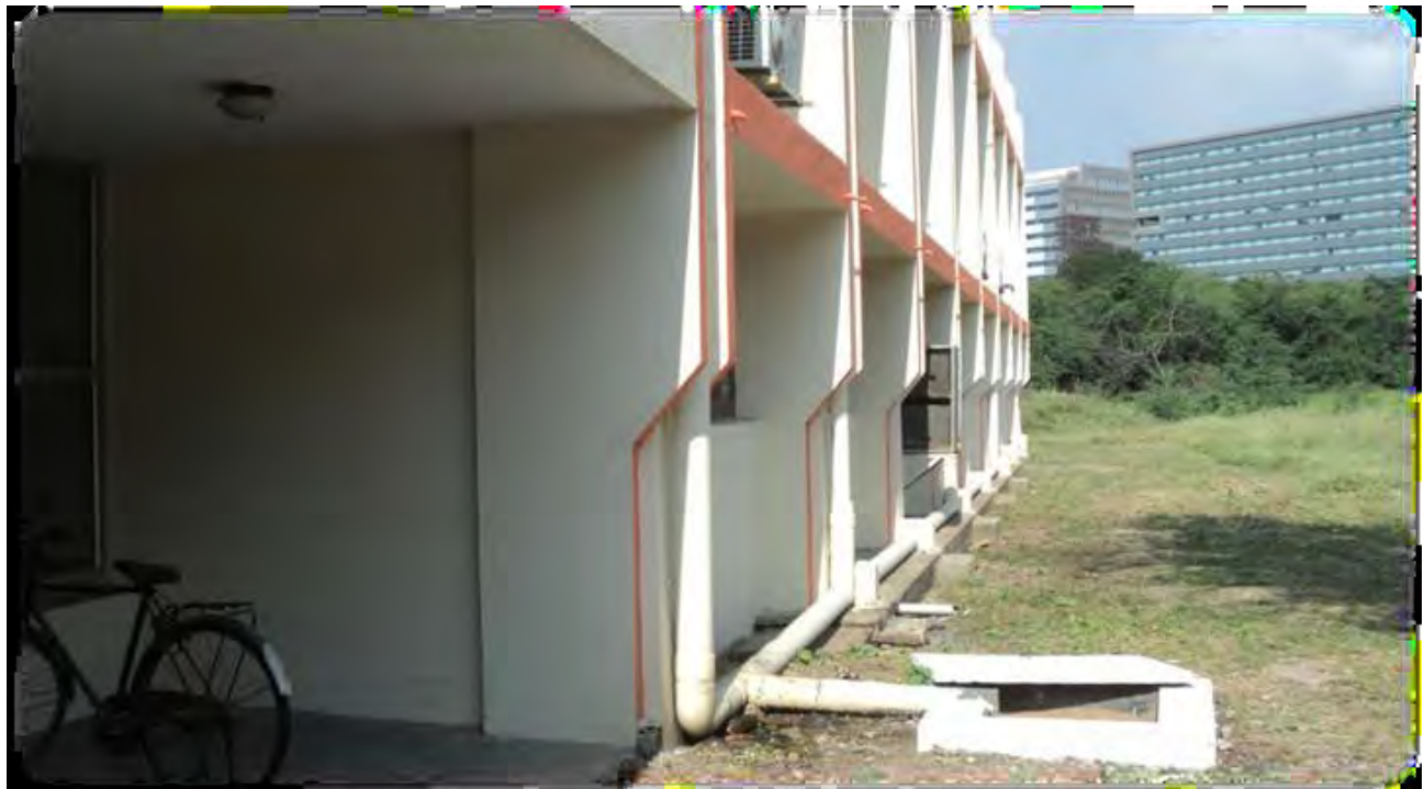
Collection, conveyance and Filtering Unit of roof top rainwater harvesting Rain water Harvesting in the premises of the NITTTR, Taramani, Chennai city, Tamil Nadu.
