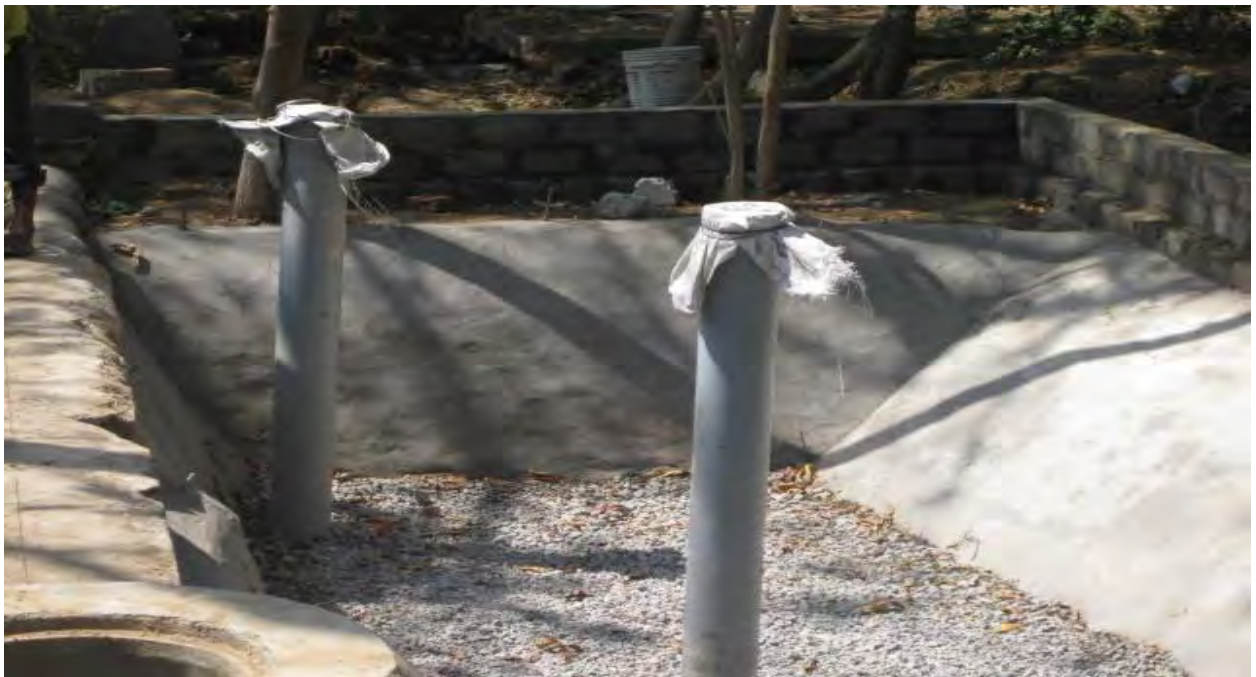
Open pond along with two recharge wells at Jawaharlal Nehru Technological University(JNTU), Kukatpaali Hyderabad, Ranga Reddy dist, Telangana
