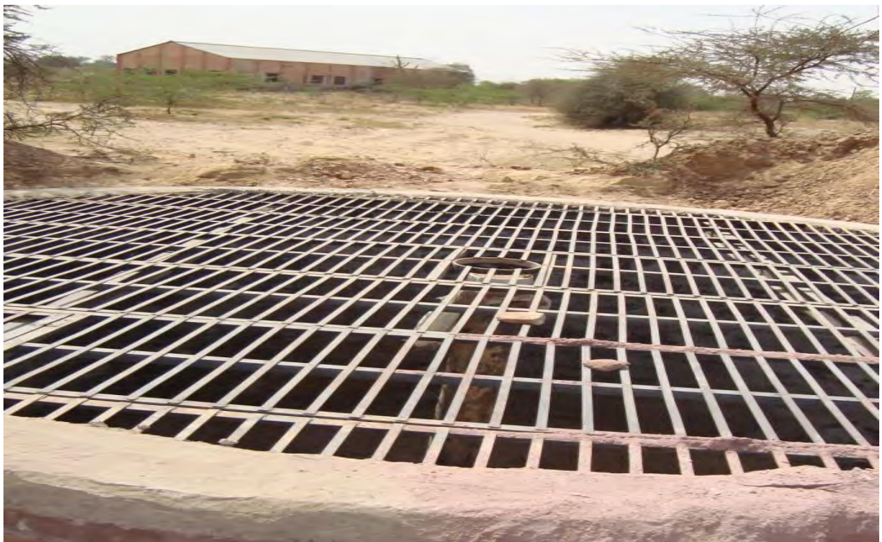
Circular Recharge Pit with filter pit & recharge tube well
