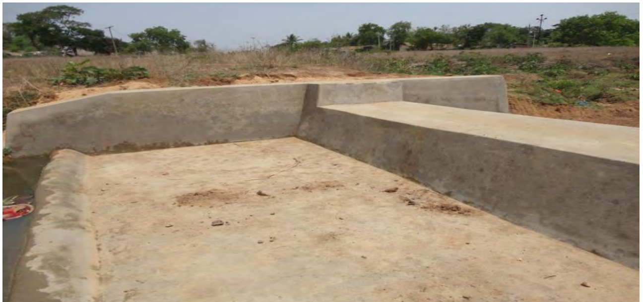
CHECK DAM OVER GANDA NALLAH Artificial Recharge Scheme for Ganada Watershed (Part), Korei block, JajpurDist, Odhisha
