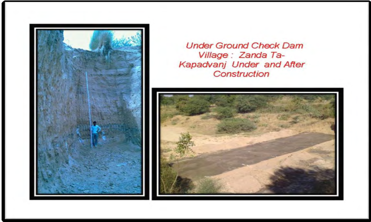
Artificial Recharge structures in Watrak Watershed, Kheda/ Sabarkantha districts
