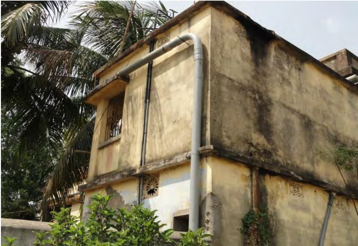
Roof Top Rain Water Harvesting Structure at Banior G.P., Nalhati-I Block, of Birbhum District
