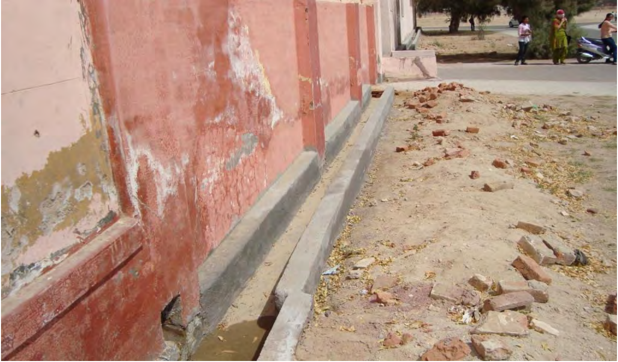
Channel for roof top run off collection Govt. Polytechnical Collage (Boys), Bikaner city, Dist Bikaner
