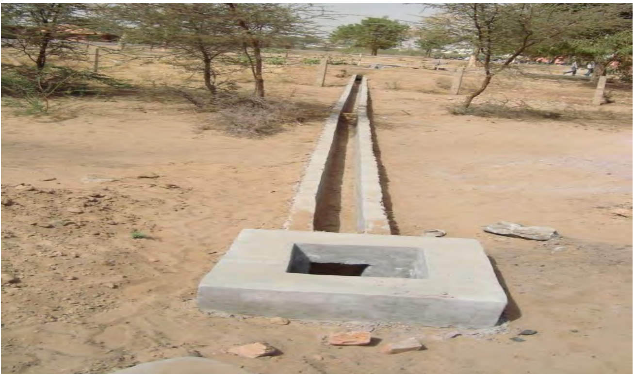
Water Channel with siphon pit-CE, IGNP Office Building, Bikaner city, Dist Bikaner
