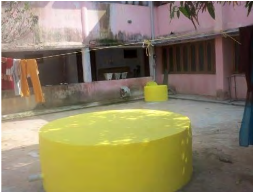
Filter Cum Collection Chamber
