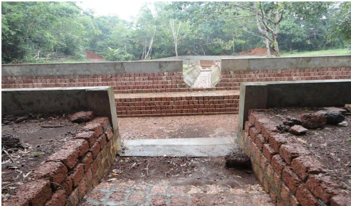
A view of Channels connecting silt tank to Recharge Pit Roof Top Rain Water Harvesting at Kendriya Vidyalaya No. 2, Vidyanagar, Kasargoddist, Kerala
