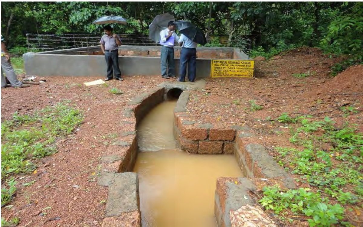
A view of water flowing through drainage channel to Recharge Pit Roof Top Rain Water Harvesting at JawaharNavodayaVidyalaya, Kanchangarh, Kasargoddist, Kerala
