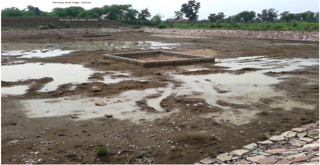
Recharge Shaft at Hathani
