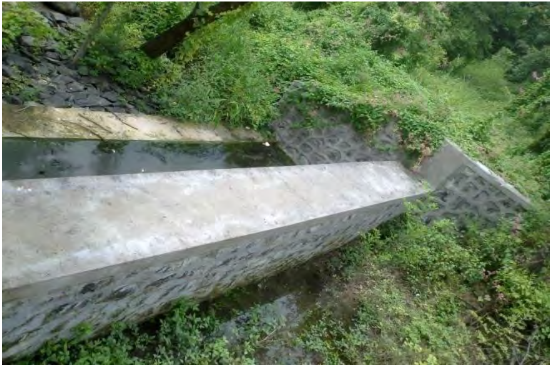
Cement Nala Bandh -After monsoon Artificial Recharge to Groundwater in Raj Bhawan area, Nagpur, Maharashtra
