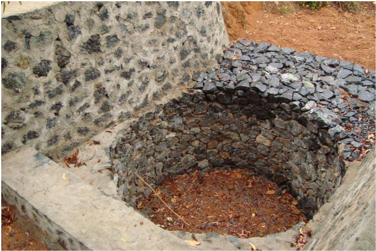
A view of the Circular Recharge Pit with out water
