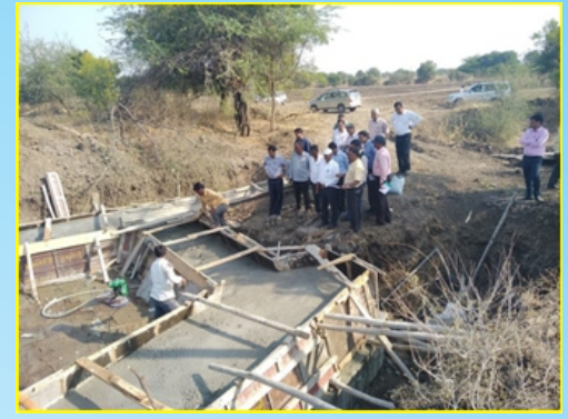
Field inspection of AR work at Kini and Khamgaon sites in Osmanabad Aspirational taluk.
