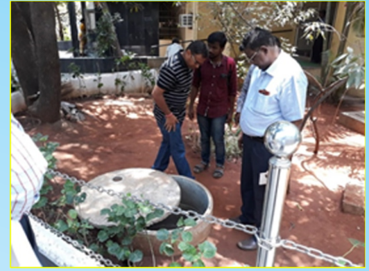
Visit of Joint Secretary, (IC & GW) DoWR, RD & GR to Rain Water Harvesting pits & wells inside Cancer institute, Adyar, Chennai on 11.05.19
