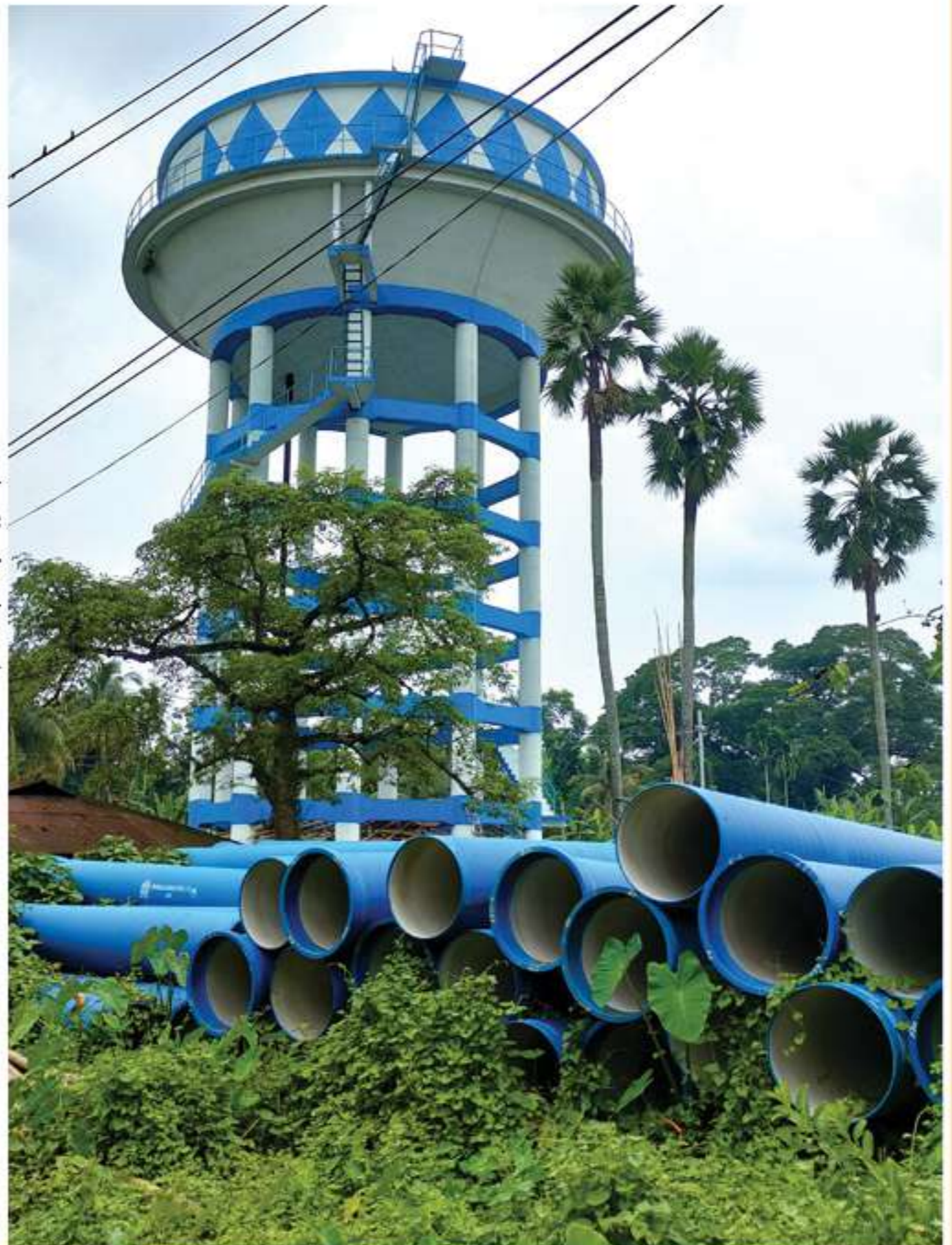
Treated Surface water supply through Pipeline
