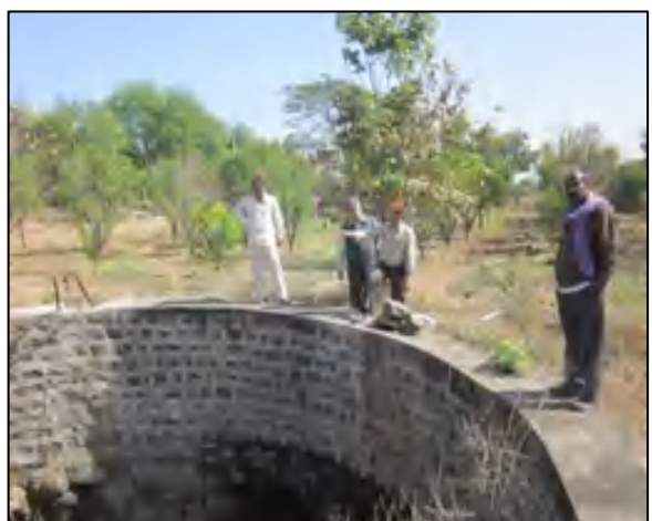
Inspection of large diameter dug well by Sh. Pradeep Dubey, Regional Director and Dr. P. K. Jain Suptg. Hg. CGWB, CR, Nagpur.
