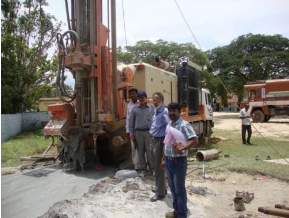
Field inspection by the Regional Director and other senior officers at Settikere EW site
