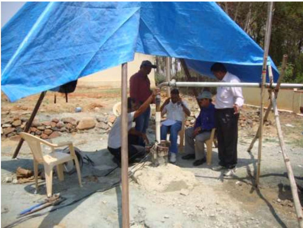
Field inspection by Region Director and other senior officers' during pumping test Sarathavalli EW site
