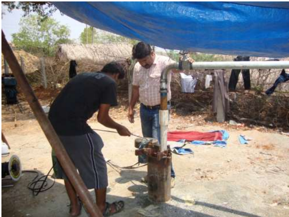
Monitoring of ground water level during pumping test at Huchanahatti EW site
