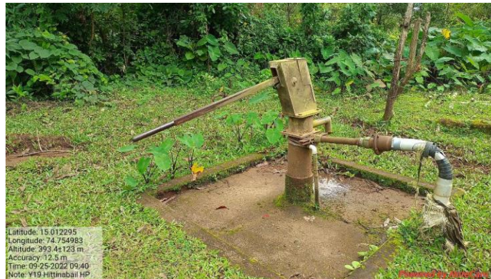
Photo 2.2: Hand pump fitted with pump in Hittanbaili (15.12295; 74.754983)
