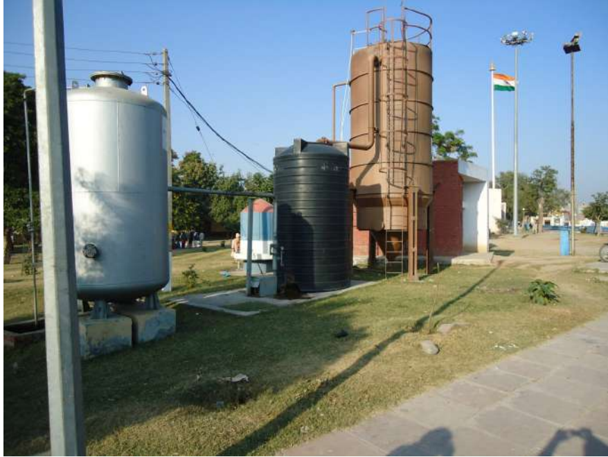
TREATMENT PLANT TO RECYCLE WATER AT SARASWATI GHAT, PEHOWA, KURUKSHETRA
