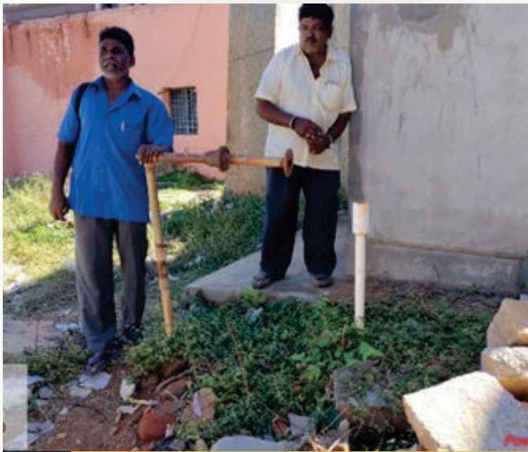
Failed BW near RO Plant, Jangamakote Village
