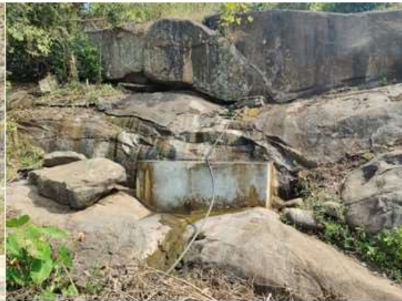
Tanks to harvest spring water under gravity, Mohana block
