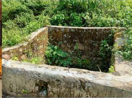
Typical well to harness the spring water, R.Udayagiri
