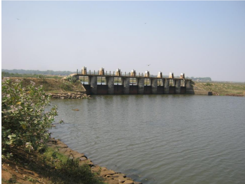
Fig.35: Sluice Gate across creek
