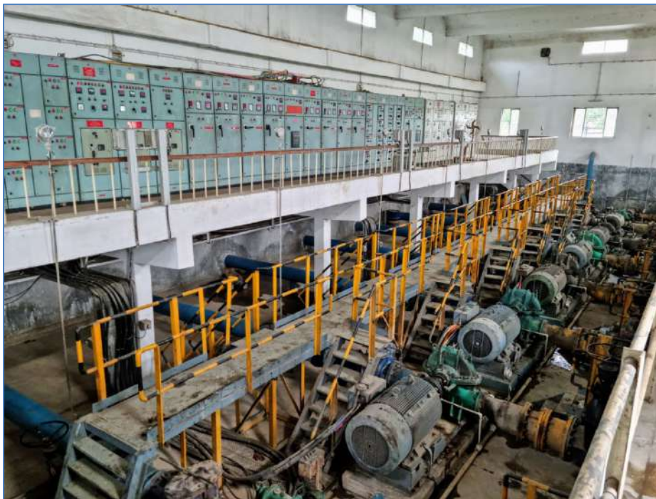
Inside view of Arsenic Removal cum Water Treatment Plant (PHED, GoWB) at Dariapur, Kaliachak-III block, Malda district
