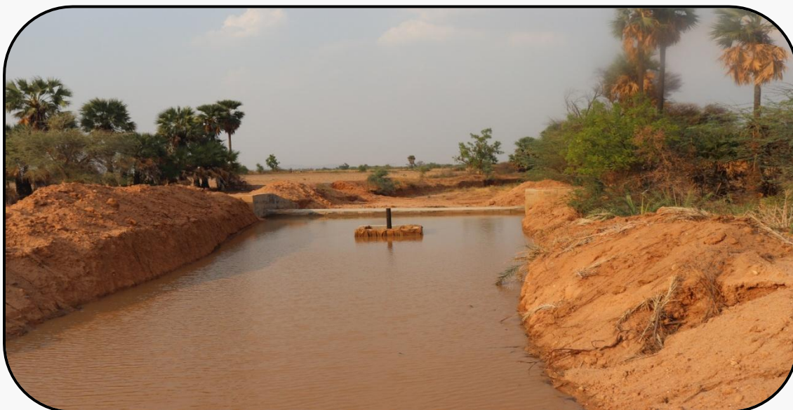
Percolation tank with Recharge shaft
