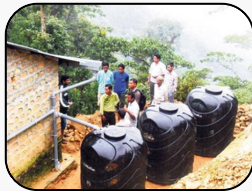
Roof Top Rainwater Harvesting
