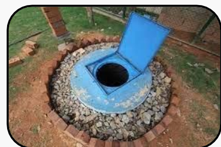
Use of drums in recharge pits
