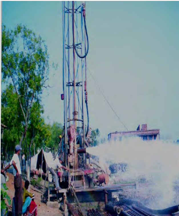
Deep exploratory Well constructed by CGWB, at Khasbalanda village, Haroa block, North 24 parganas district, West Bengal using cement sealing techniques
