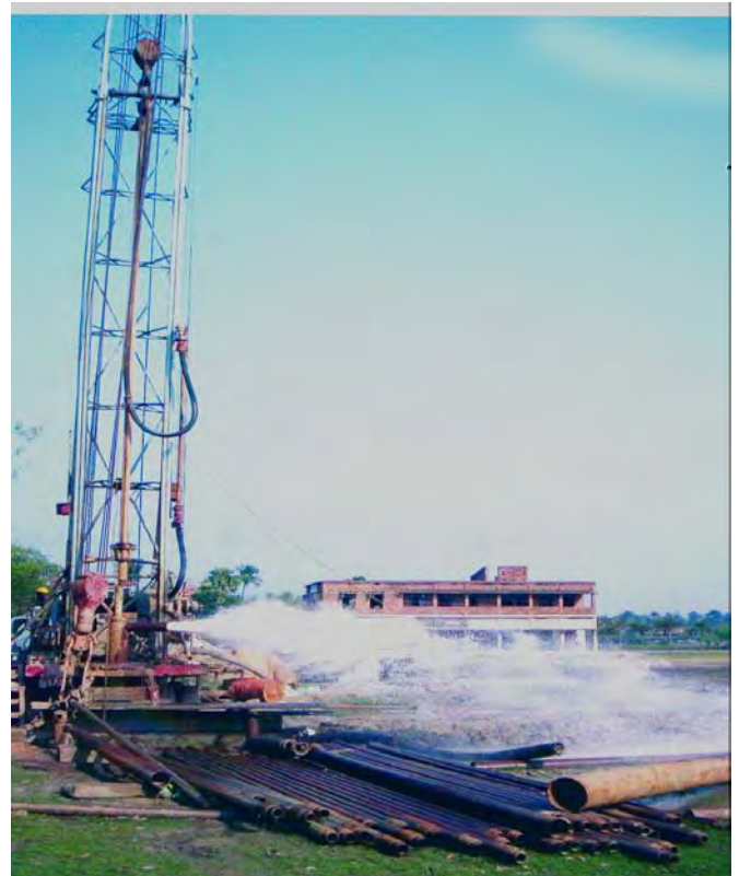
Deep exploratory Well constructed by CGWB, at Khasbalanda village, Haroa block, North 24 parganas district, West Bengal using cement sealing techniques ( cement sealing depth 100 to 105 m bgl ) tapping the deeper arsenic free aquifer (175 to 205 m bgl) yielding 34 lps of arsenic free water.
