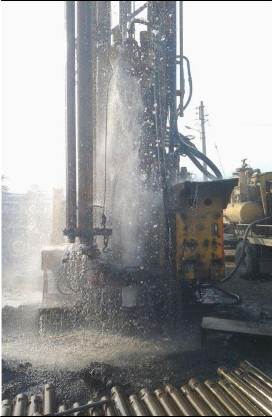
Fig 2.2 Ground Water Exploration at Pilot Project in Chandrabhaga Watershed, Nagpur District (AQMAH) District
