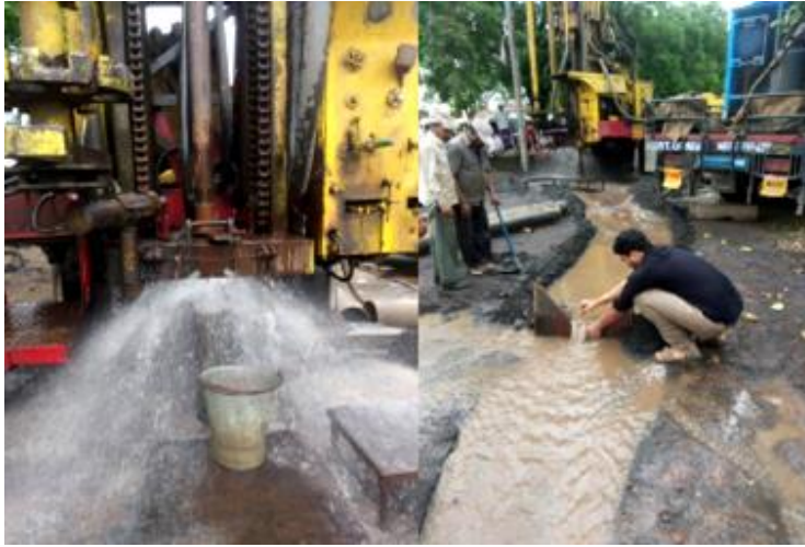
Fig.3.5: EW drilled down to a depth of 185.50 m bgl at Taroda village in the Wardha taluka of Wardha district, Maharashtra state yielded a discharge of 465 lpm
