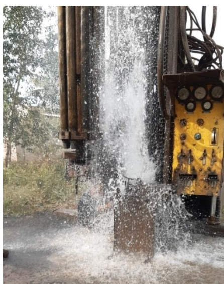
Fig. 3.1 EW at Samarth gaon village in Satara taluka of Satara district, Maharashtra with discharge of 731 lpm
