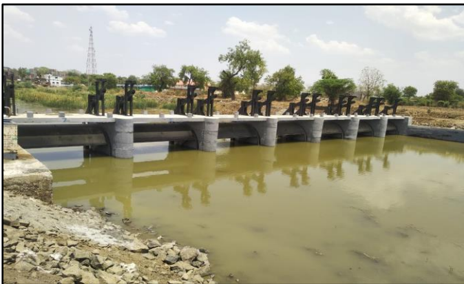
Tiwasa (Gates in open position)
