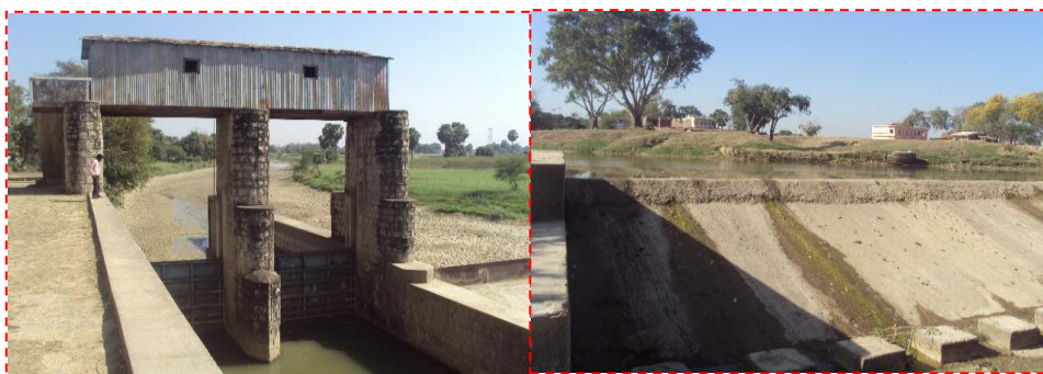
Plate 4: (a) Small barrage on the river Kasma, from which a small canal (also known as Pyne) goes for irrigation (west to the photograph). (b) Check dam on the river Ramrekha on way from Amba to Deo, still makes a small reservoir in the month of February, assuring irrigation for the adjoining agricultural lands.
