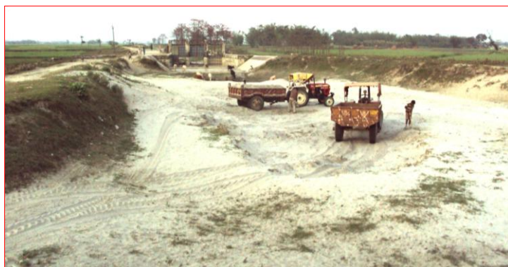
Figure 5: High siltation in canals of Kosi command area in Supaul district. The image showing de-siltation work.
