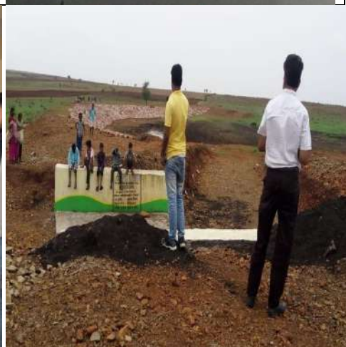
Artificial Recharge structure, Prithwipura.
