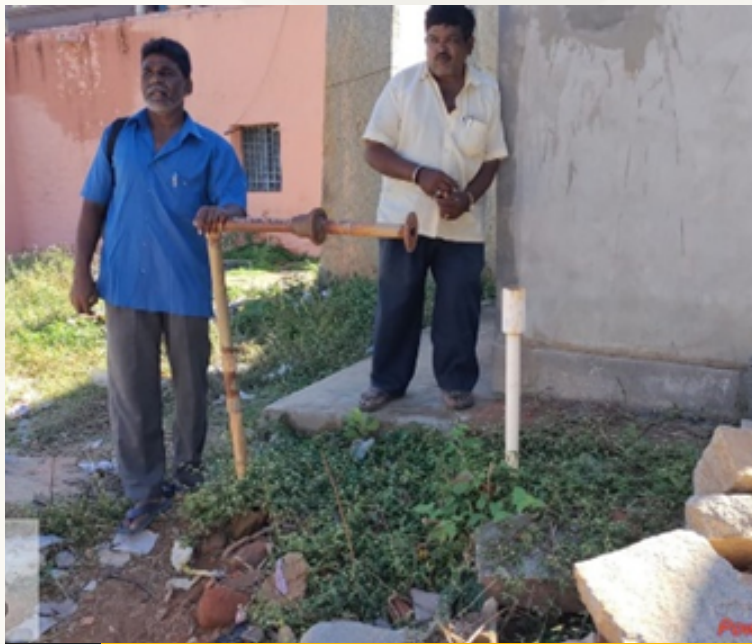
Failed BW near RO Plant, Jangamakote Village
