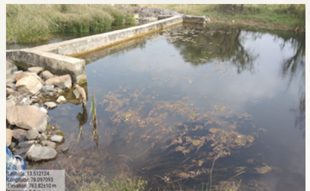
Damaged CD in Chintamani Taluk
